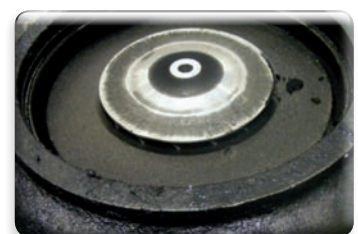
Compressor end oil leakage
